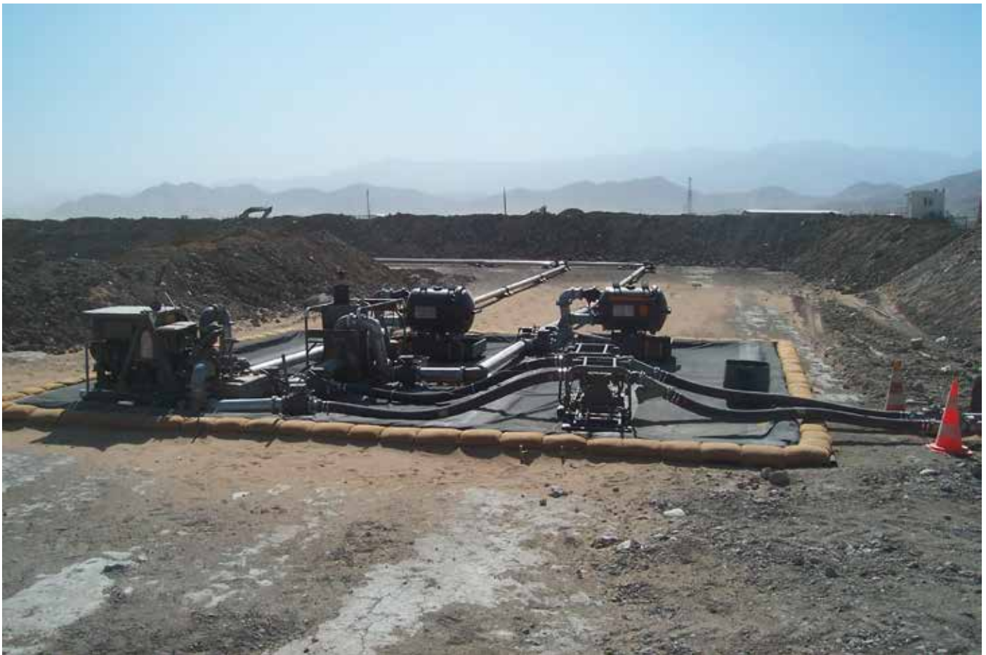
Typical setup of pump unit, filter water separator and bulk flow metering
